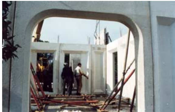
A residential project in the North of Iran - Erection of the panels- looking inside
